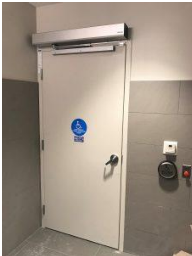
Figure 3: A restroom with a door opener and push button (Limitless Automatics & Doors, n.d.).
